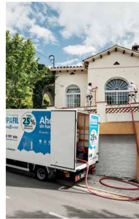
SUPAFIL being installed at a home in Spain through the outside, meaning minimum disturbance to the homeowners.
